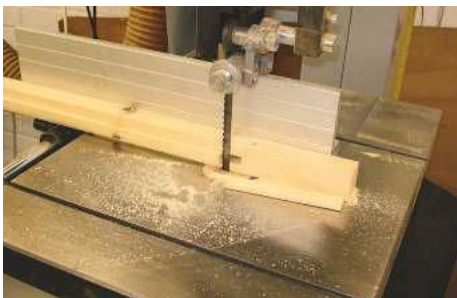
▲ Pic.16 The bottom of the top stiles and the top of the bottom are left over length to allow 'joggles'
